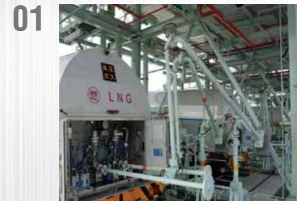
01 Loading Arm for tank lorry
