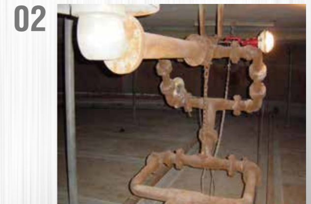
02 Roof Drainage System
